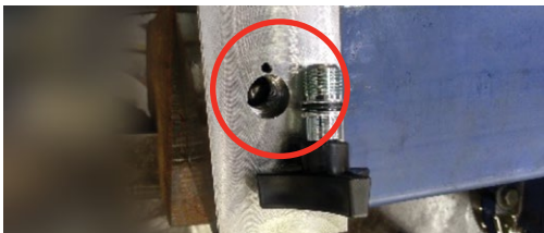
Figure 4: Control valve removed. Note large ball visible in control valve port.
